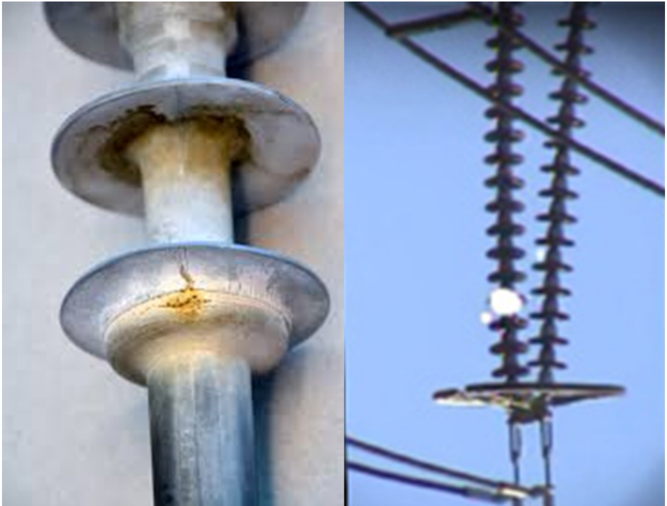
Figure 8. Degradation Insulators using corona camera.
