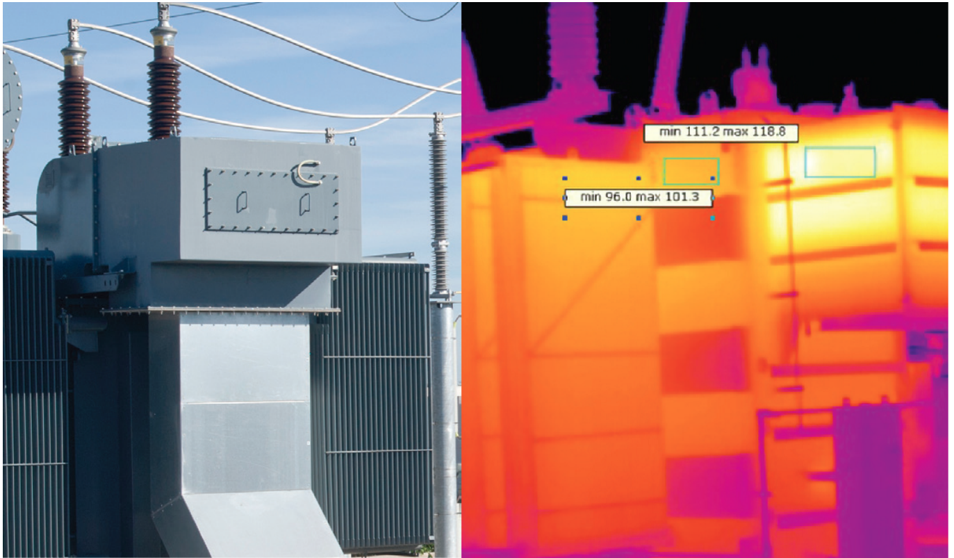
Figure 7. LTC inspections using IR camera.
