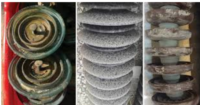
Figure 11. Cracked porcelain Insulators.
