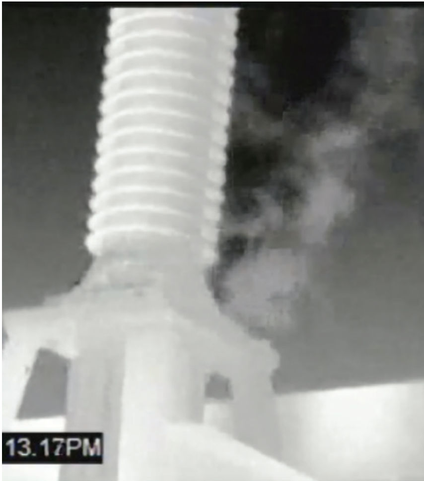
Figure 5. SF6 Circuit Breakers using IR camera
